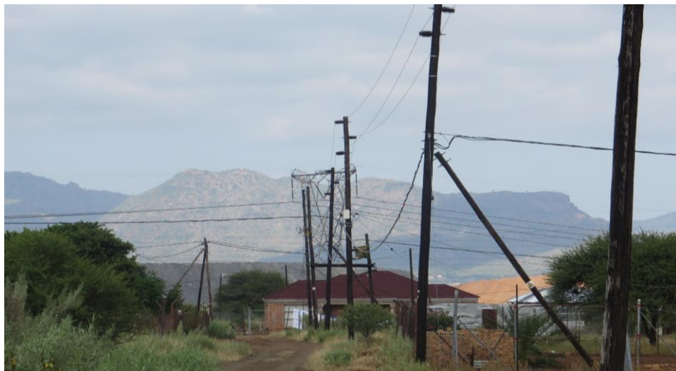
Above: Electrical poles and a transformer installation at Manyaka village.
