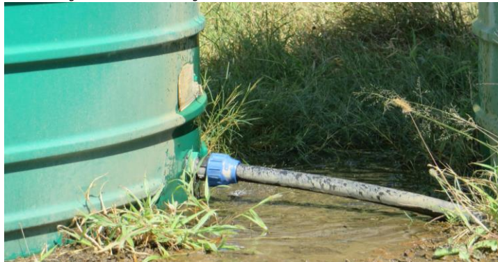
Below: A large leak on the lower Anglo JoJo tanks
